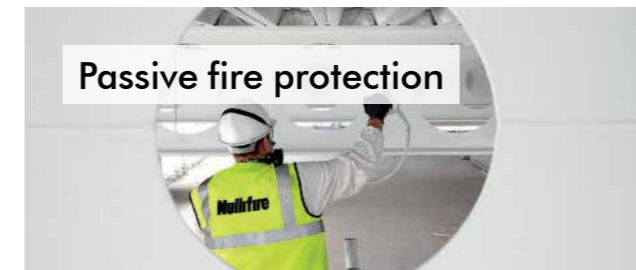
Intumescent Coatings, Fire Stopping
