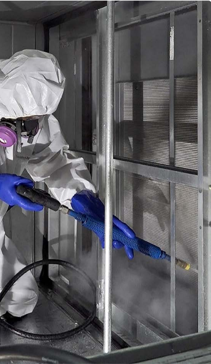
Pure Air helps facilities disinfect their HVAC systems with high temperature steam to restore airflow and energy efficiency while also improving air quality.
